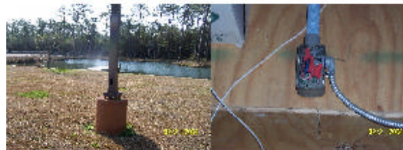
Sample areas of missing covers
