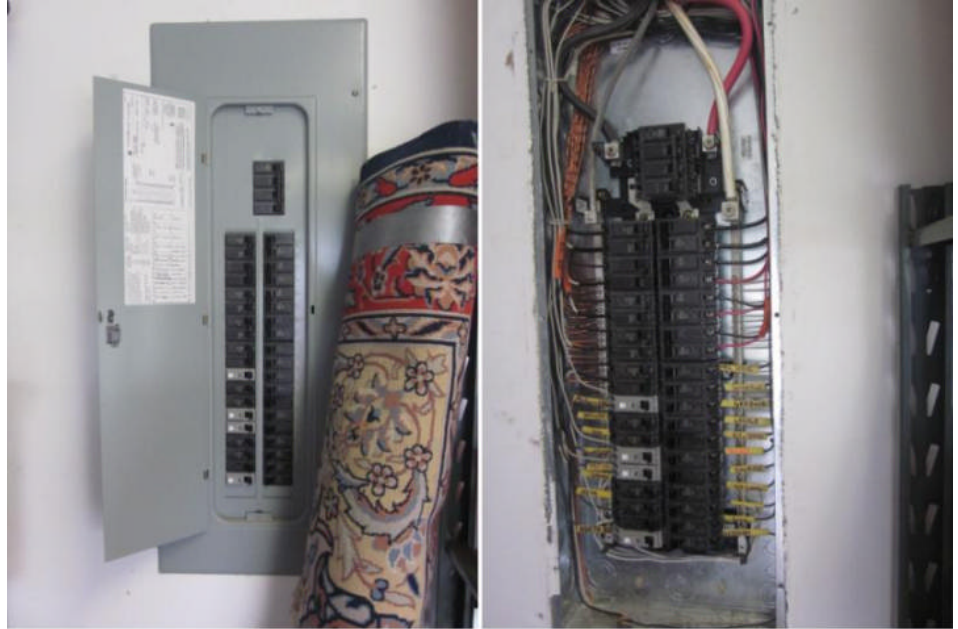
Circuit and wire sizing correct so far as visible
