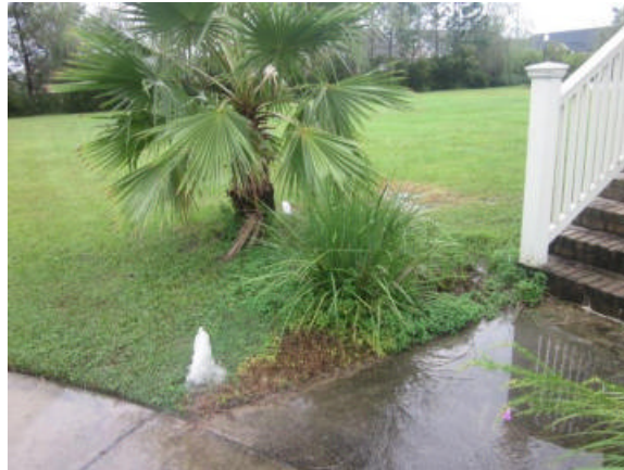
Heads are broken and I could not get enough water flow to test the sprinkler system.
