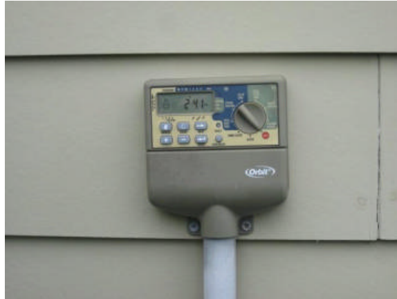
The timer is located on the exterior wall and is functioning properly at this time.
